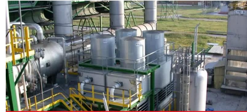
Cooling System Failures in Industrial Equipment: Summer Troubleshooting Guide
